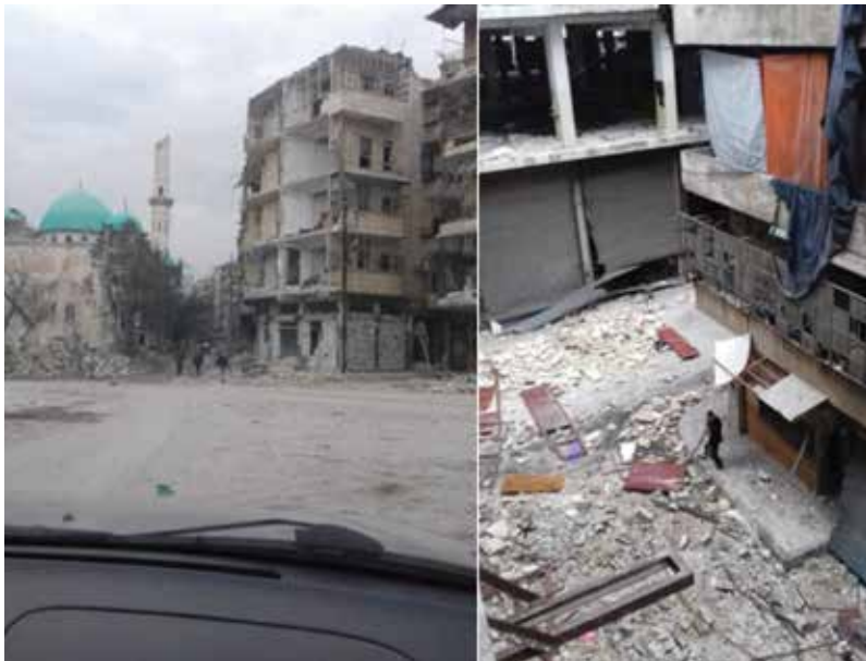
Figure 20: 16 December 2016 Photos from Aleppo. Karm al-Qaterji Main Roads are Passable, but Smaller Roads Still Contained Debris at the Time 45
