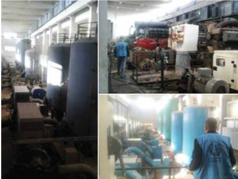
Figure 32: Bab al-Nayrab Water Pumping Station: Partially Damaged, Partially Functioning
