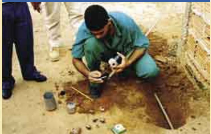
Installation of micro-meter in household connection, Parauapebas
