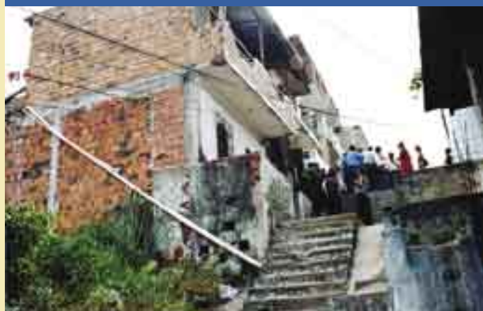
Steep Change of Condominial Branch Level (pipe attached to wall), Sao Caetano, Salvador de Bahia
