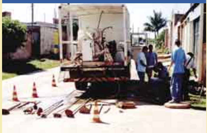
Maintenance Equipment for Condominal Branches, Brasilia
