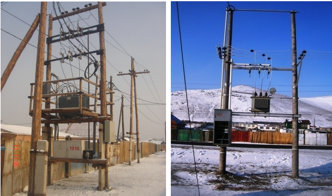
Rehabilitated transformers substation with wooden and concrete poles in ger areas
