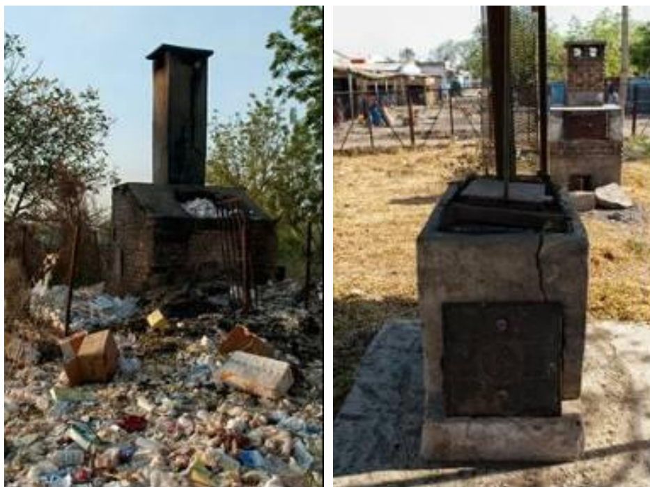
Figure 6-17: Old and broken incinerators, Malakal
