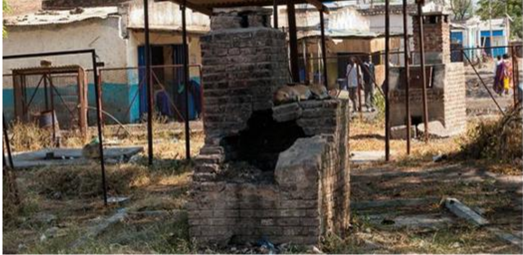
Figure 2-2: Old Medical Waste Incinerator, Malakal
