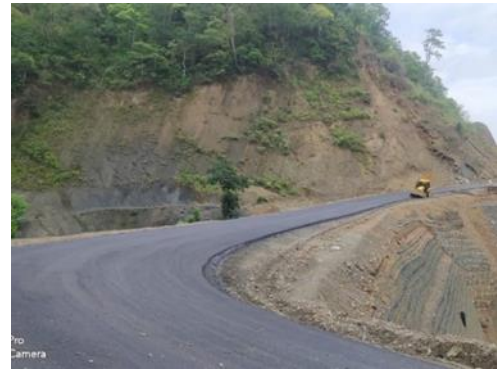
Box Culvert with High Embankment Geo Cells and GeoGrids at Ch: 21+745 km
