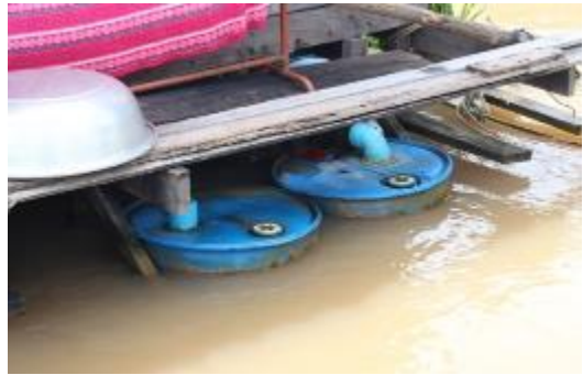
HandyPod treatment system installed under a floating house. Source: Wetlands Work
