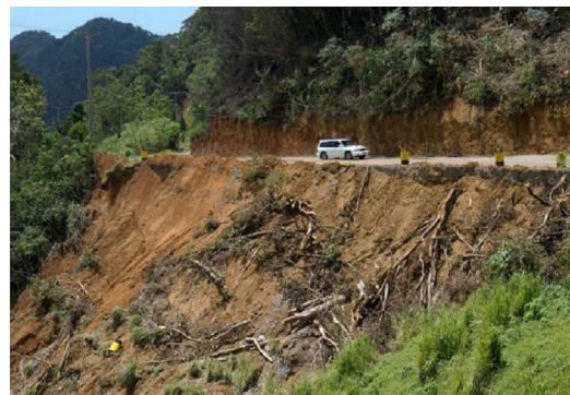
Major landslide on Imperial Highway
