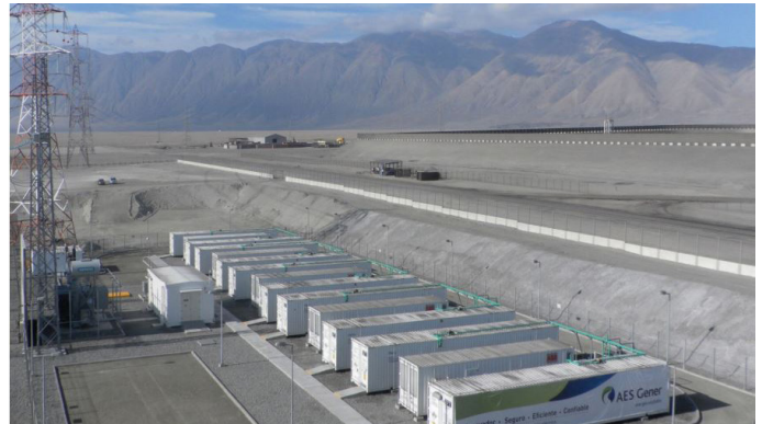
Picture 4.1 Lithium Ion Battery Containers at the AES Angamos Plant in Chile
