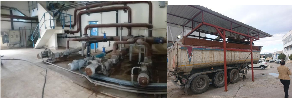
Figure I-12: Sludge Drying Unit
