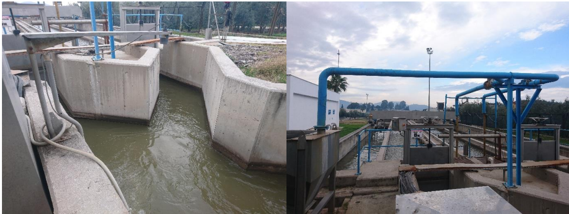
Figure I-3: Inlet Structure & Screen
