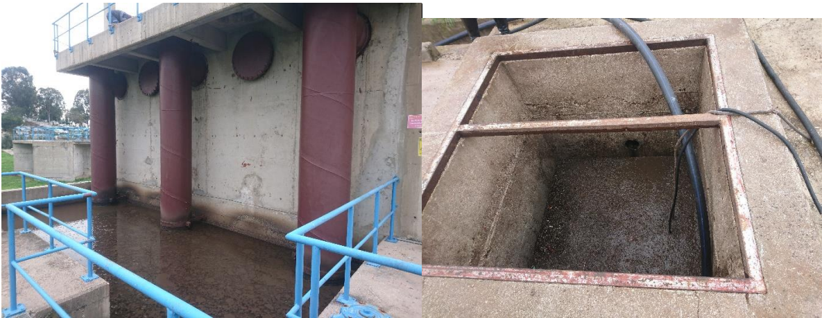
Figure I-7: Sludge Transfer Tank
