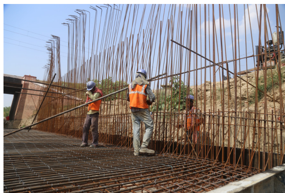
The World Bank is financing India's Eastern Dedicated Freight Corridor where electrified railway lines will reduce GHG emissions by 2.25 times over 30 years. Environment friendly transportation is being piloted in five cities, and a multimodal project is working to link India's north east with Bangladesh and Myanmar.
