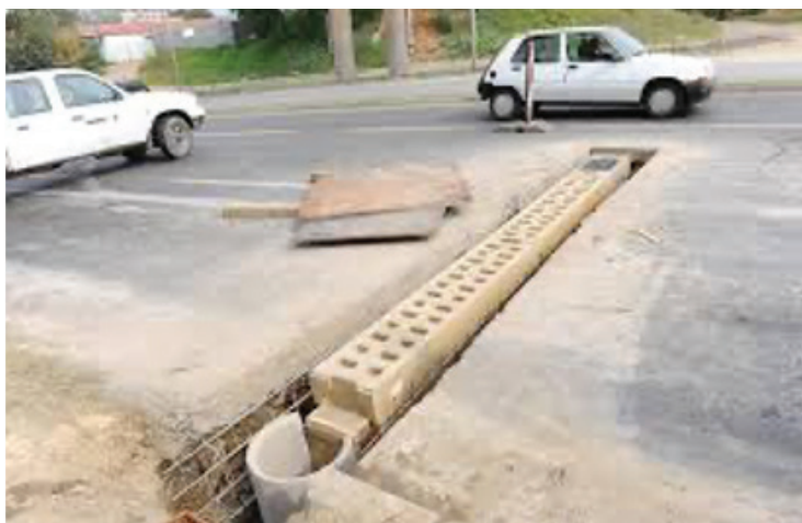
Photo 2. Reconstruction of atmospheric sewage on Boulevard Kiro Gligorov in the City of Skopje. (Photo credit: Plusinfo.mk, October 15, 2014.)
