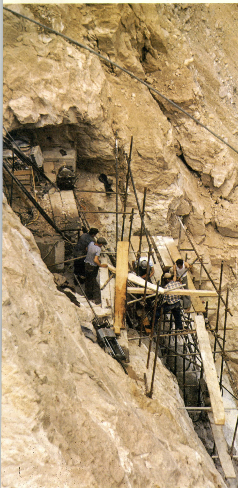
Detail Shows Tough Building Conditions from the Sites of One Hydro Power Plant at the River Neretva in Hercegovina
