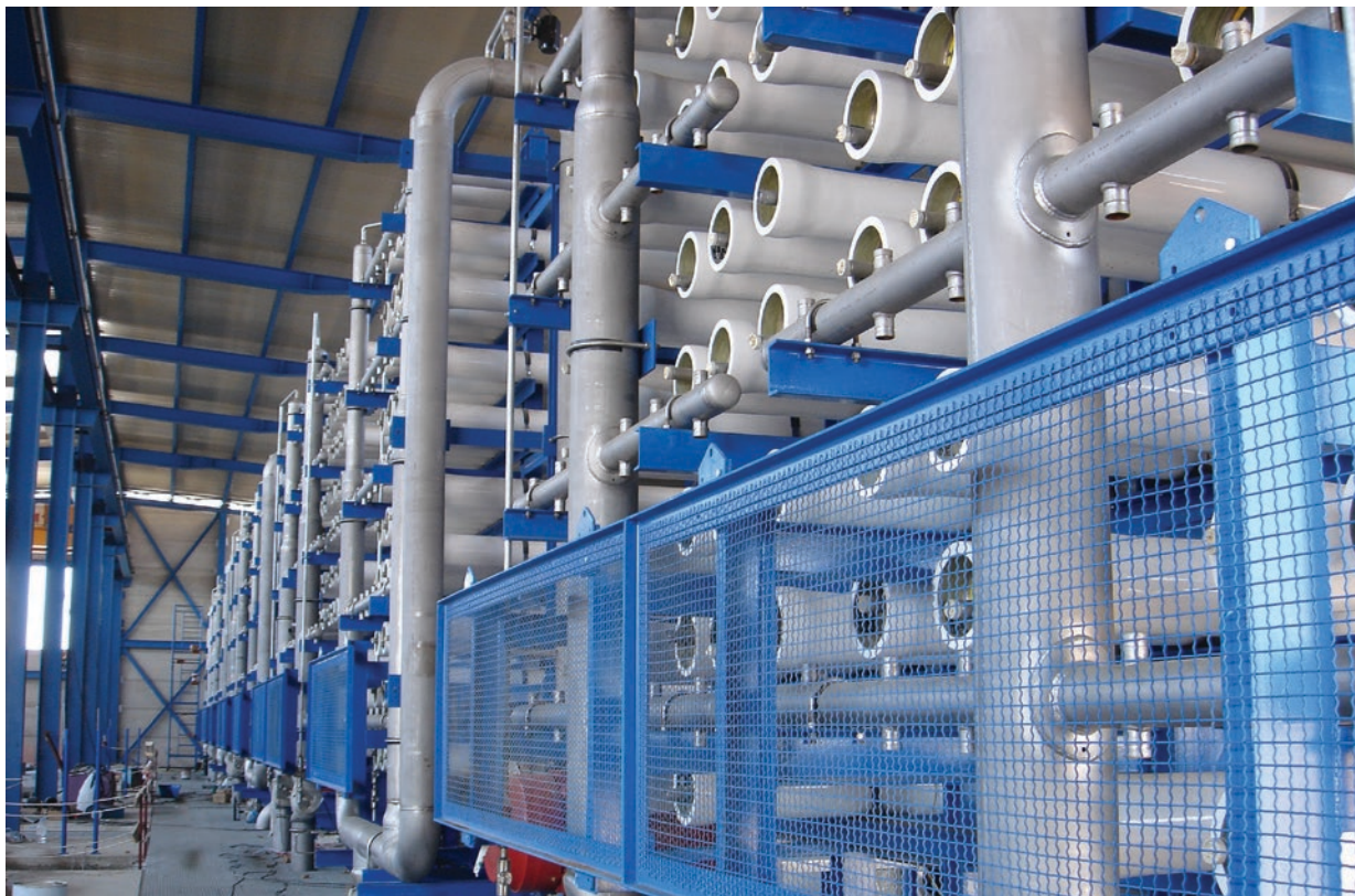
PHOTOGRAPH 3.6. Desalination Plant in Almería, Spain
