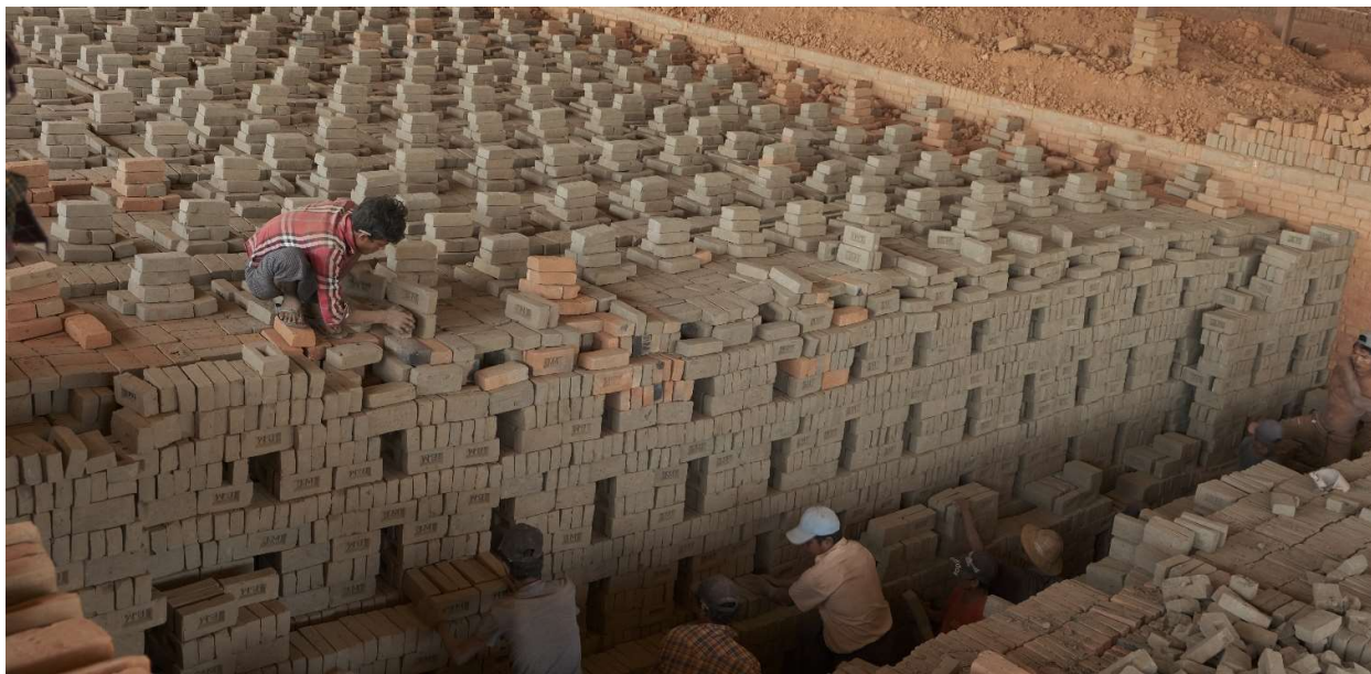
Figure 84 - Workers laying raw bricks in a Hoffman kiln as fire is progressing towards them
