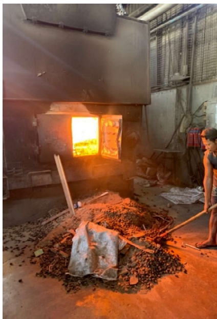
Figure 21 – Manual feeding, solid fuel boiler at Hong Kong vermicelli factory, Yangon
