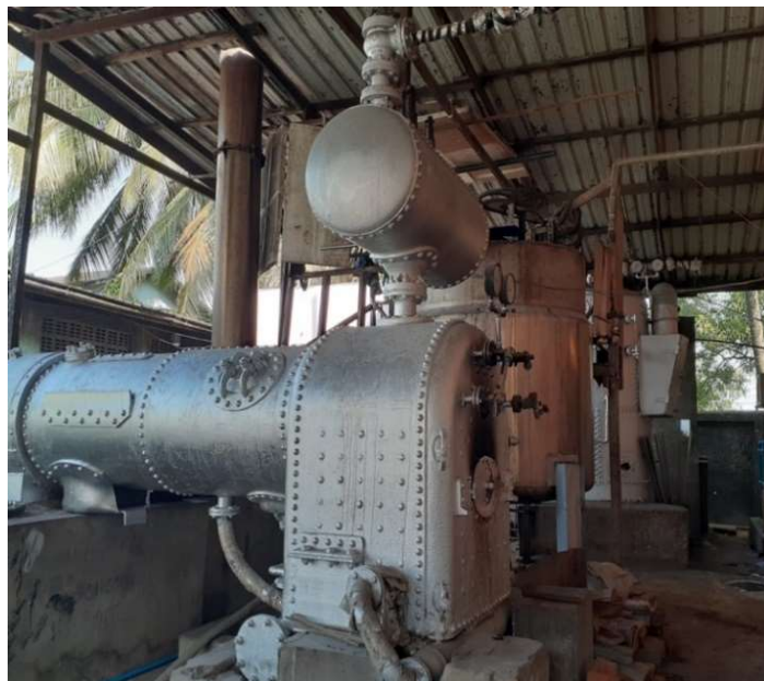
Figure 22 – Wood-fired vertical boiler at Eagle Brand Chilli Sauce factory, Yangon
