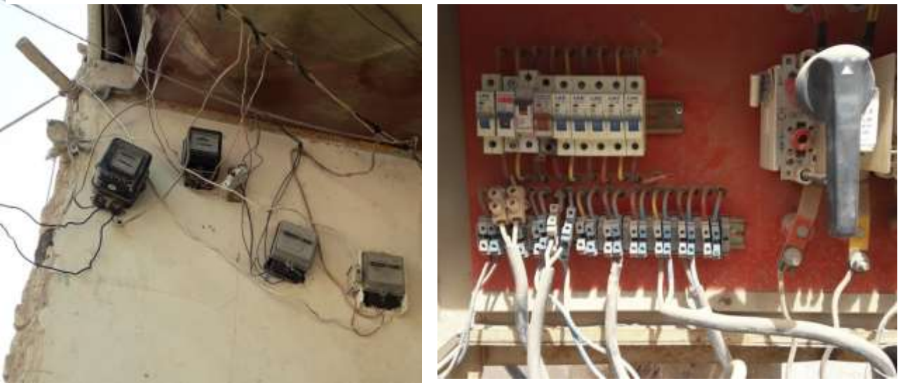
Figure 115 Wiring and meters
