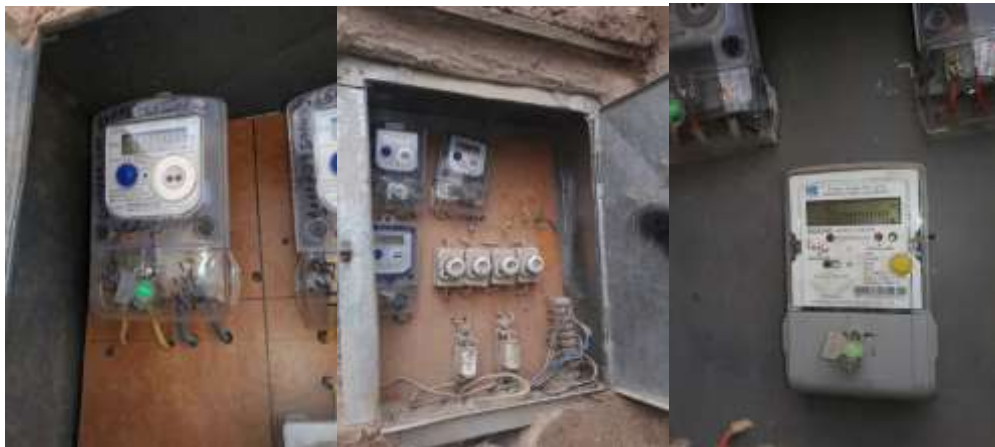
Figure 58 Different sets of electricity meters administered by DABS
