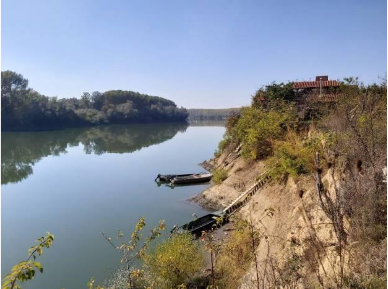
Picture 5. Residential houses and most significant damages to the river bank along the project section
