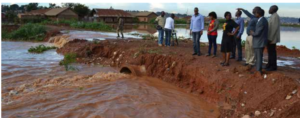
Lubigi channel - City planners at work to provide drainage in the city. Sheila Gashishiri (2013)
