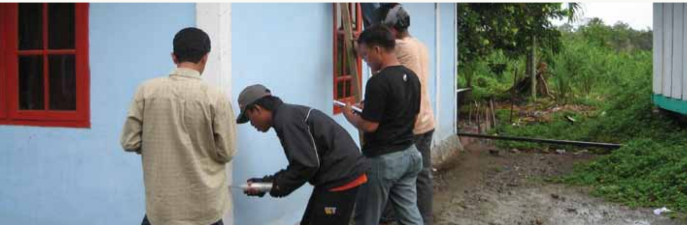
Rekompak facilitators test the side and upper beam of the house walls to ensure the strength. Lasikin village, Aceh, 2009.
