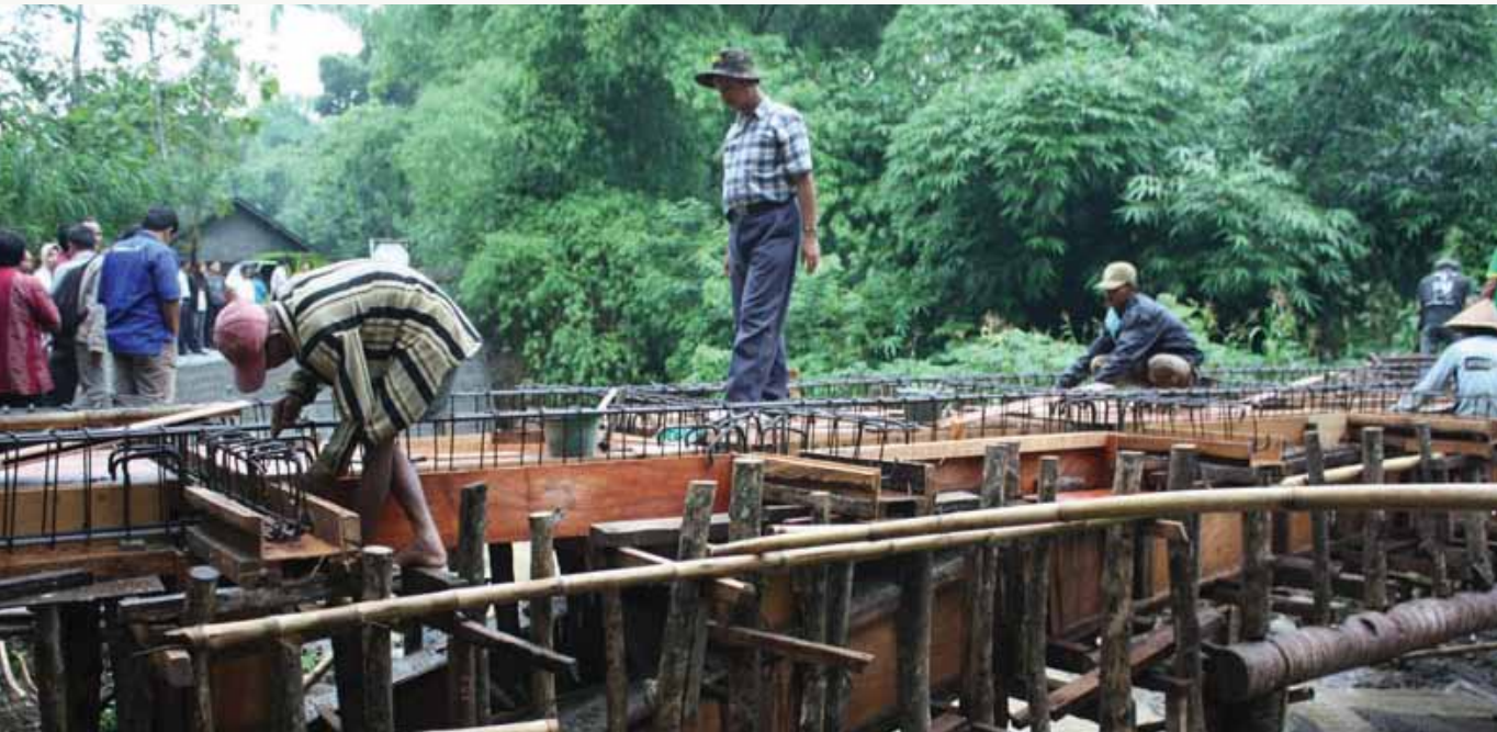
A facilitator inspects the quality of the construction of this bridge in Gayamharjo, Sleman.
