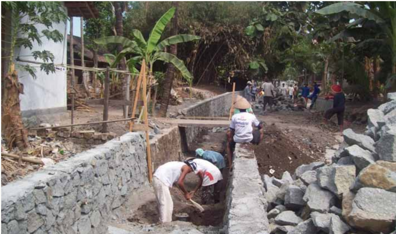
A new drainage system is being constructed to prevent flooding in Wonokromo, Bantul, in the Yogyakarta Special Region. Projects such as this were identified through a community planning process under Rekompak.
