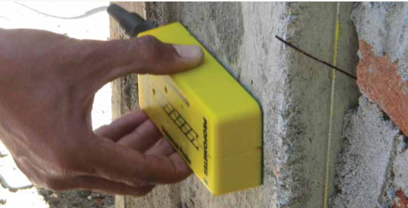
Facilitator measure the strength of the house beam in Lasikin village, Aceh.
