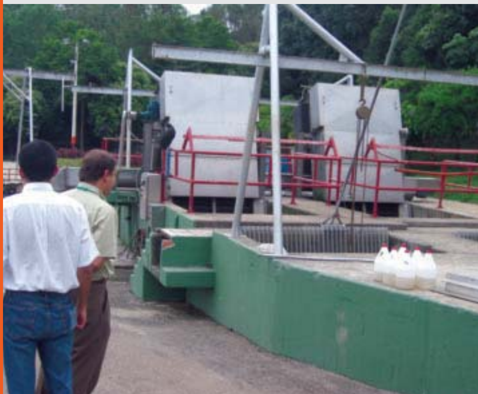
Improvements in the existing wastewater treatment plant are designed for the elimination of methane.
