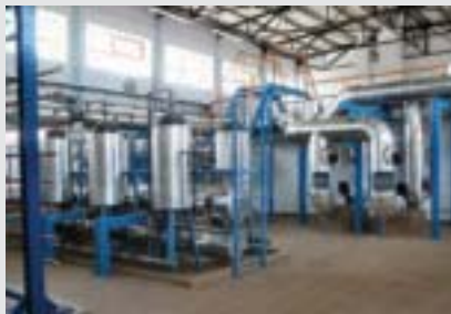
Geothermal heat production facilities at Stargard.
