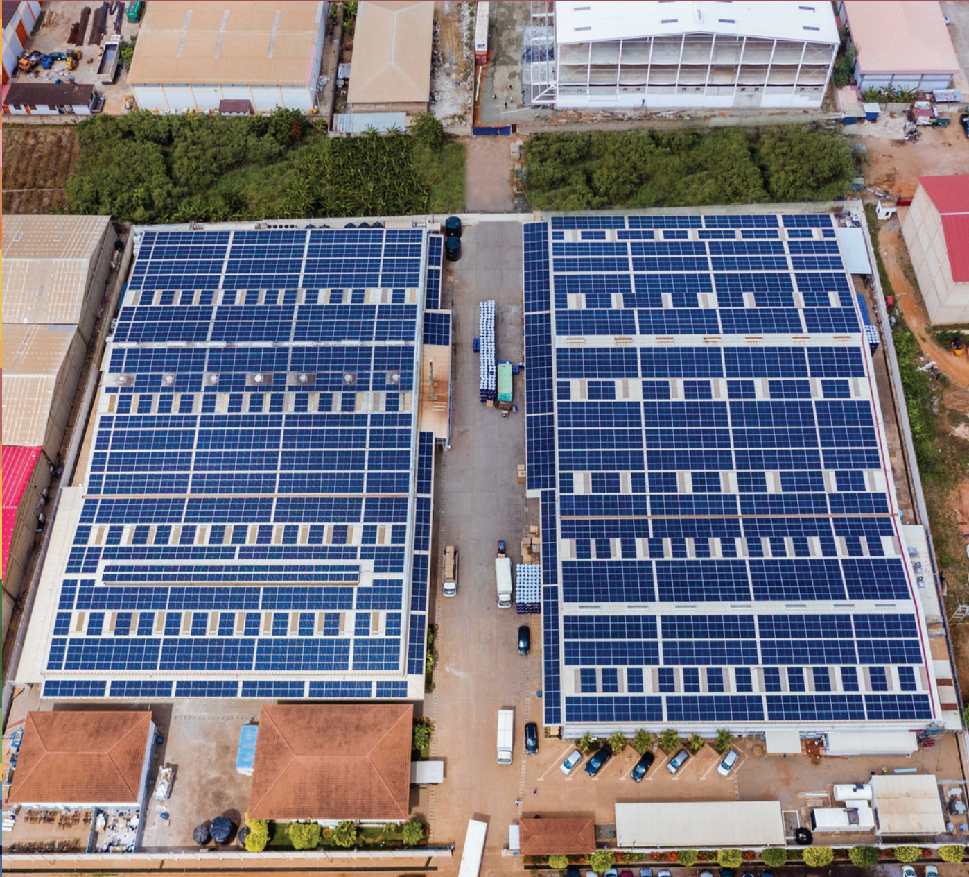
Rooftop solar generation at Chandour Cosmetics Ltd in Accra, Ghana. Photo: © Ghandour
