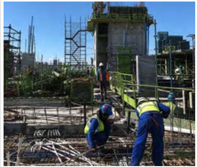
Construction workers working on laying pipes in construction area in South Africa. Photo: © wilpant.
