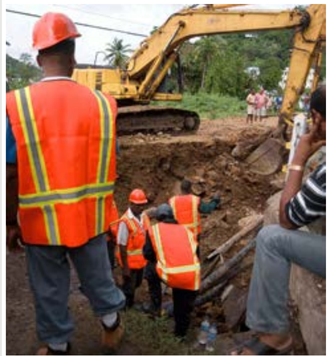
Workers in St. Lucia repairing damaged bridge from Hurricane Tomas. Photo: © jaminwell.
