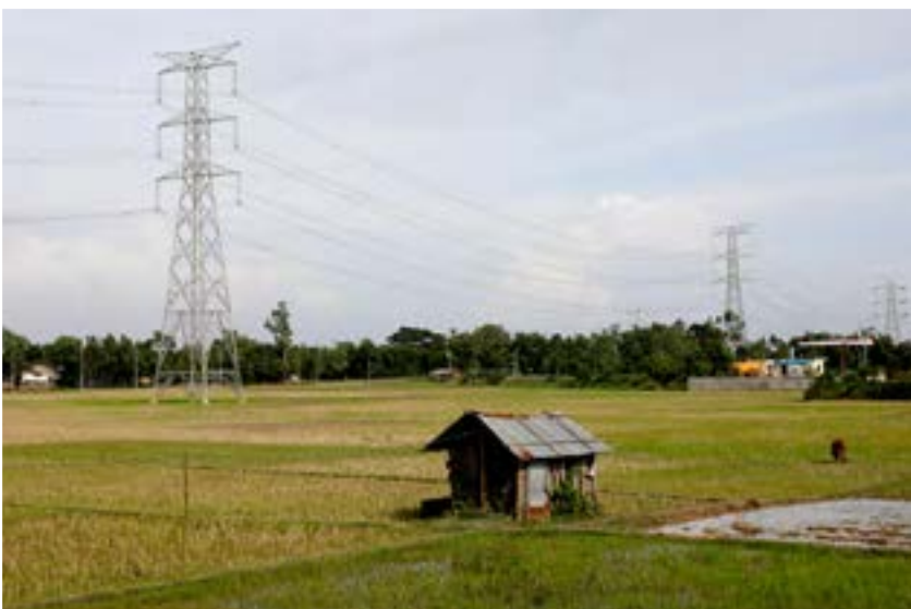
High voltage electric transmission line in rural Bangladesh. Photo: © Md Golam Mortuza Ali.
