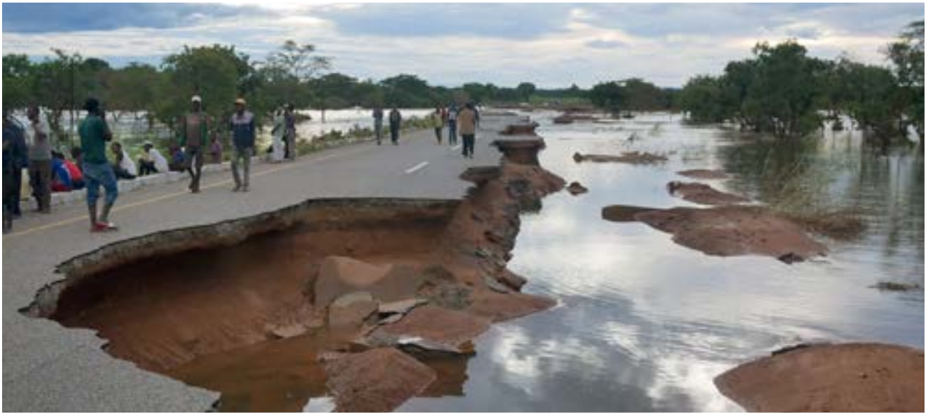
Mandimba villagers wait for help at a collapsed bridge after Cyclone Freddy. Photo: © Roy Gilham.
