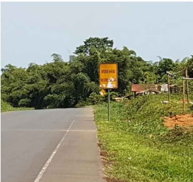
FIGURE A4.18: EXAMPLE OF PAVEMENT MARKINGS AND ROAD SIGN CONDITIONS ON TRADITIONAL CONTRACT
