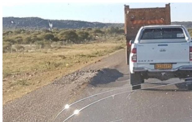
FIGURE A4.44: PAVEMENT DEFECT ON ROAD MAINTAINED UNDER TRADITIONAL MAINTENANCE CONTRACT
