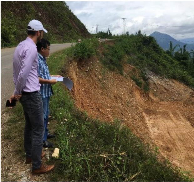
FIGURE A4.11: EXAMPLE OF SLOPE STABILITY ISSUES ON HIGHWAY 16B
