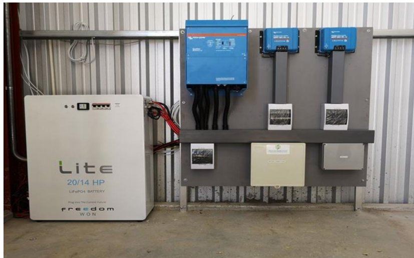
Figure 8: A solar ESS hybrid site in South Africa with Freedom Won Battery
