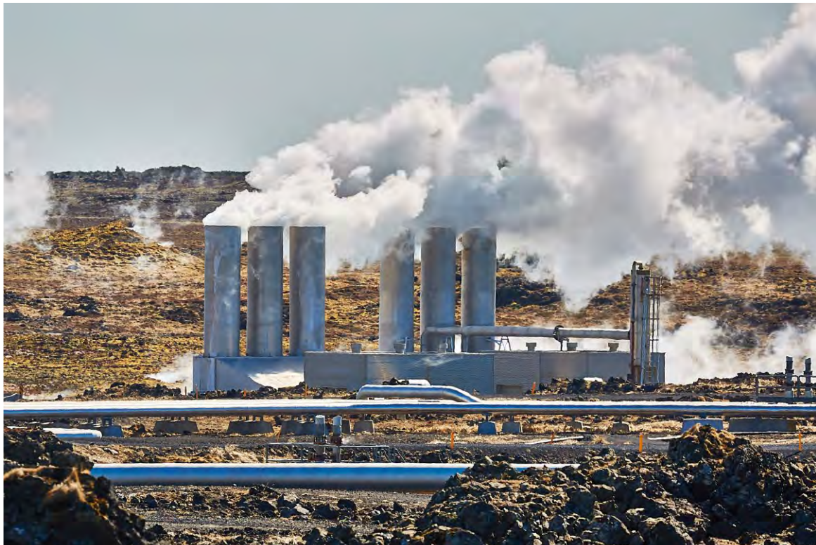
Photo: Geothermal power plant
