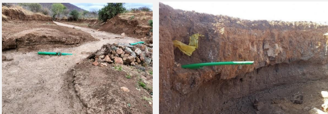
Figure 3.1. Fiber damage from seasonal pluvial flash floods
