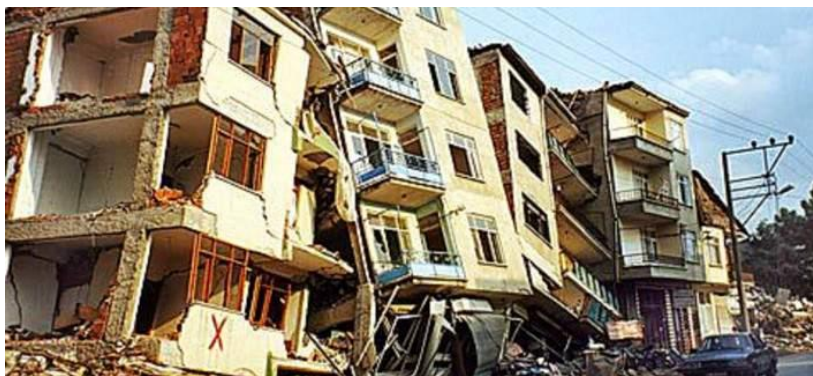
Figure 8: Damage to buildings in Kalamata 1986 earthquake
