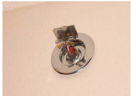
Figure 37. Side wall sprinkler
