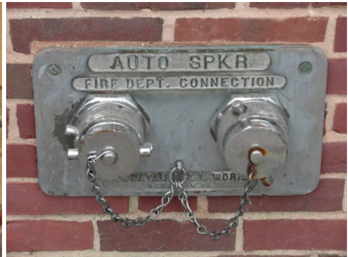
Figure 32. Exterior connection to sprinkler system
