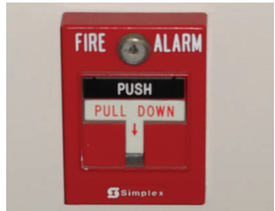
Figure 25. Manual fire alarm station
