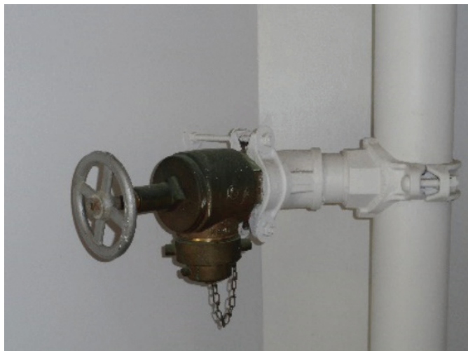
Figure 32. Exterior connection to sprinkler system
