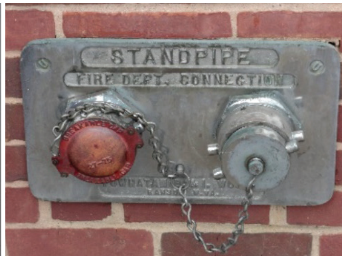
Figure 33. Interior hydrant/standpipe valve and hose connection
