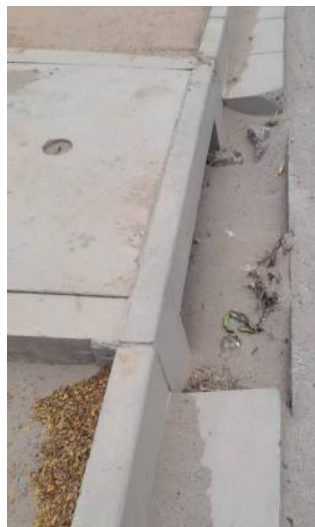
Photo 7: Loose soil in the entrance of manhole
