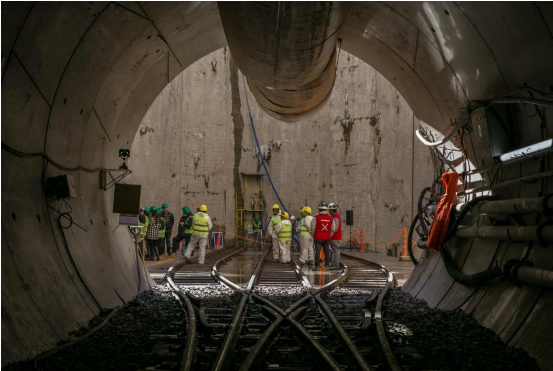
Vega drainage tunnel, with its 8.4 kilometers long and more than 5,3 meters in diameter. Source: https://buenosaires.gov.ar/compromisos/23000-metros-de-obras-hidraulicas-y-sistema-de-alerta-de-tormentas
