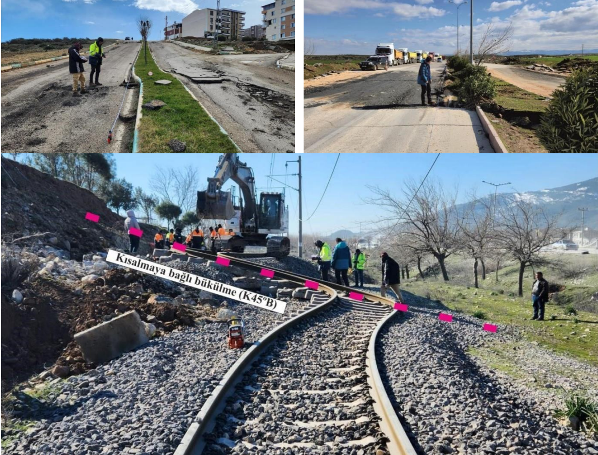
Figure 10: Examples of visible surface ruptures along roads and railways captured during field investigations in southeastern Türkiye. Source: MTA (2023).
