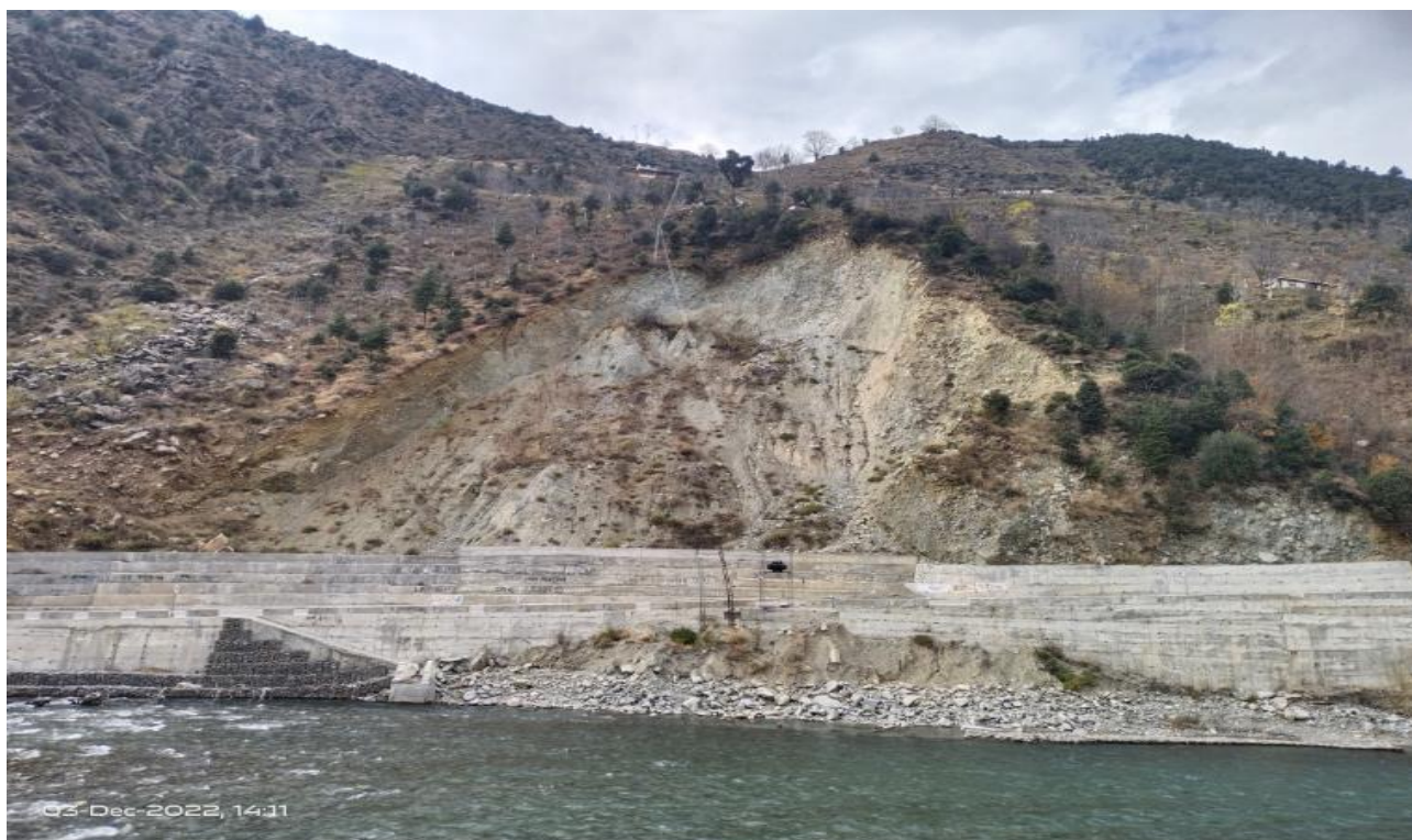
Figure 5-11: Landslide along weir Location 2 at Right Bank
