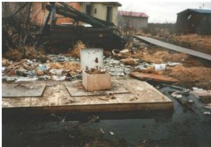
Photo A.1 Underground Communal Wastewater Tank, Alaska
