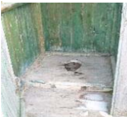
Photo 3.7 Pit Latrine with Improved Slab
