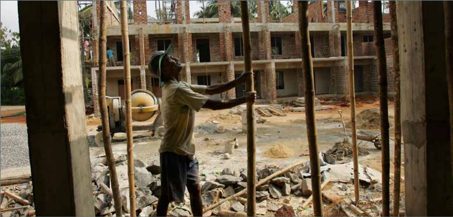
A Sri Lankan construction worker builds a new school, to replace one destroyed by the Tsunami, December 27, 2005 in Galle, Sri Lanka. Photo credit: Paula Bronstein
