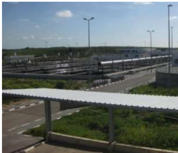
Figure 12-33: Basins for activated sludge on the left side
