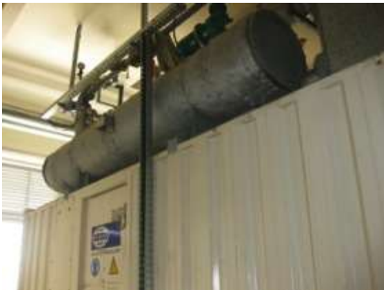
Figure 12-24: Containerised diesel gen-set
