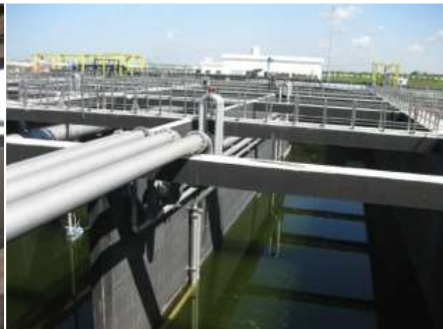
Figure 12-37: Sludge activating basin (1 of 3)
