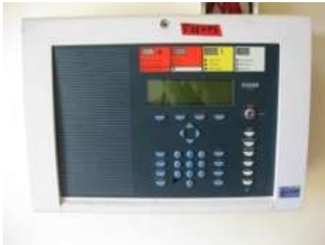
Figure 12-29: Fire detection unit
