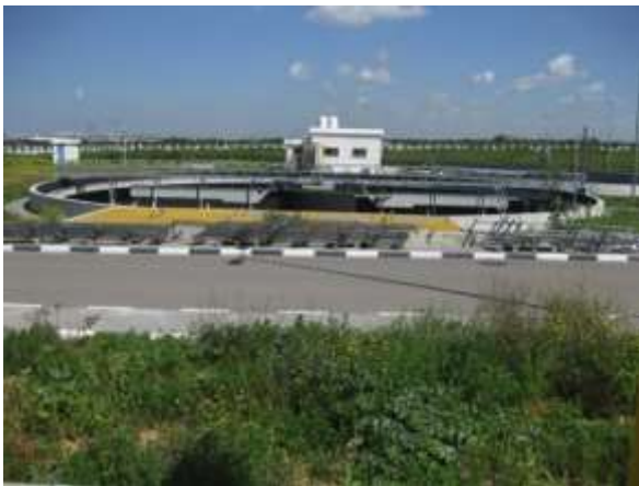
Figure 12-40: Final clarifier (1 of 3)
