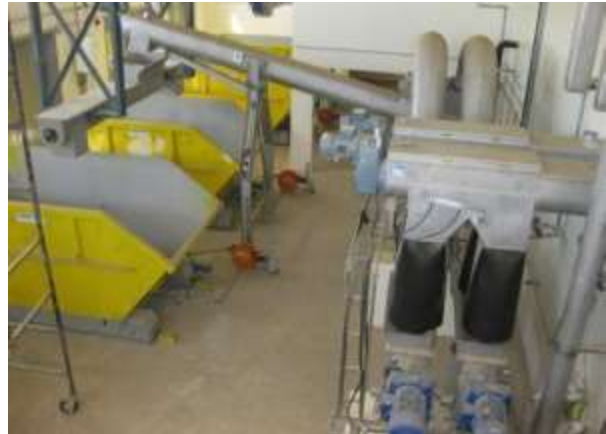
Figure 12-39: Sand washing zone
