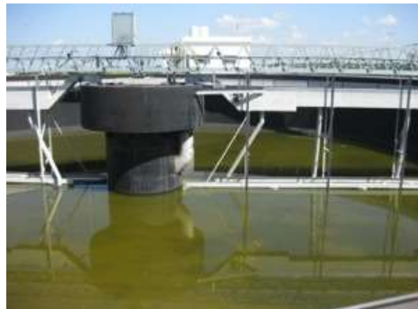
Figure 12-41: Final clarifier (1 of 3)
