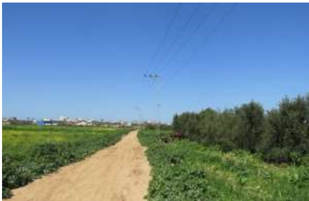
Figure 12-17: OHL feeder from Jibaliya
