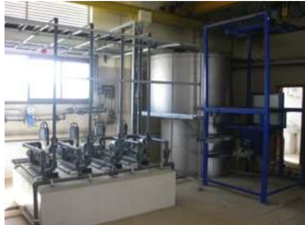
Figure 12-35: Sludge silos and sludge dewatering building – screw pumps for sludge
