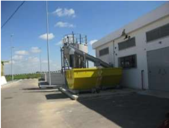
Figure 12-34: Sludge silos and sludge dewatering building – outside equipment
