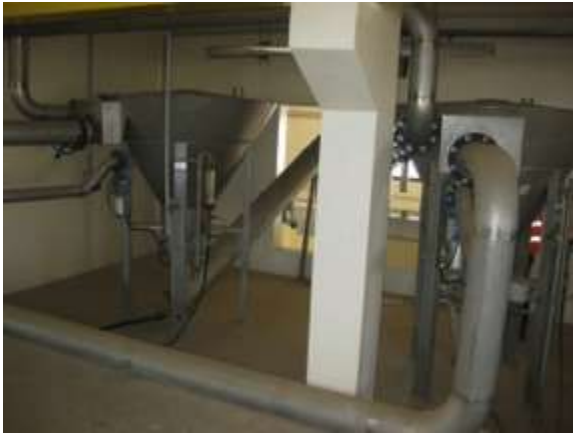
Figure 12-38: Sand washing zone
