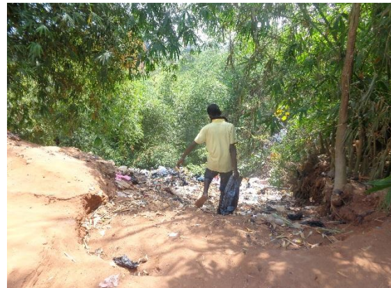
Figure 18 Residents dumping refuse at erosion site
