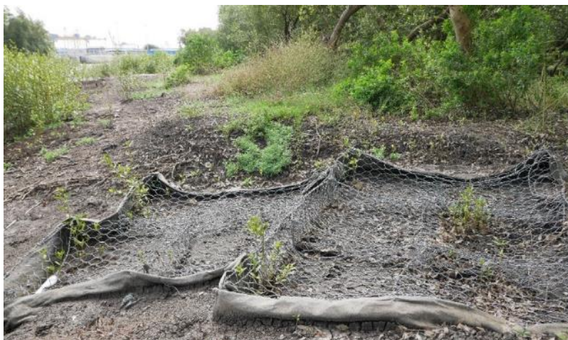
Figure 3-5 Gabion baskets subject to theft of stones (Basin 1)
