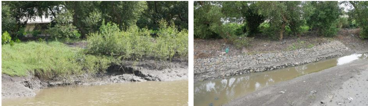
Figure 3-4 Failure of river slope in Basin 1, slipped gabion mats in Basin 3
