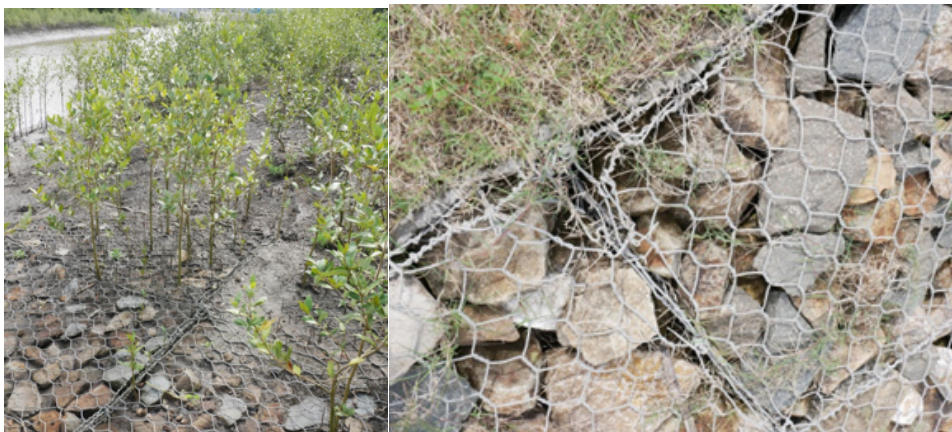
Figure 3-11 Mangroves establishing in the gabion baskets (left), grass growing over gabion baskets (right). July 2018
