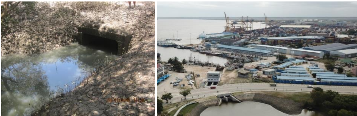
Figure 3-9 Old outlet culvert in 2012 (left) and new tidal outlet structure in 2018 (right)
