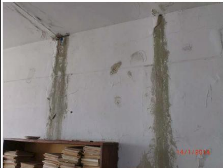
Main building 2. floor, Office with cracks on wall and ceiling (Bathroom 2)
