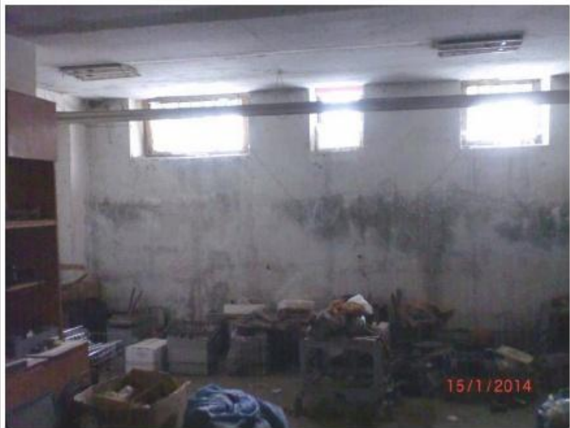
Main building basement, Workshop room street side with a damp external wall (Liquid Volume V3)
