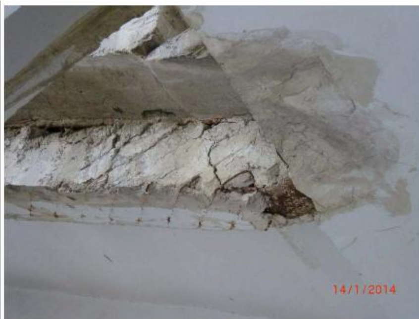
Main building 2. floor, Stairwell south side with damage on the staircase
