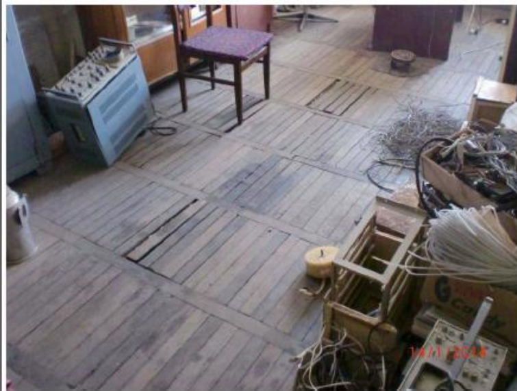
Main building 2. floor, Office with damage to the floor covering (Bathroom 2)
