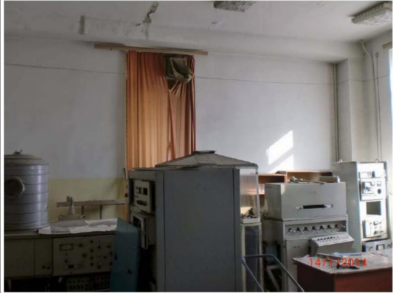
Main building 1. floor, Large laboratory room with flaking on the ceiling and beams (Force F)
