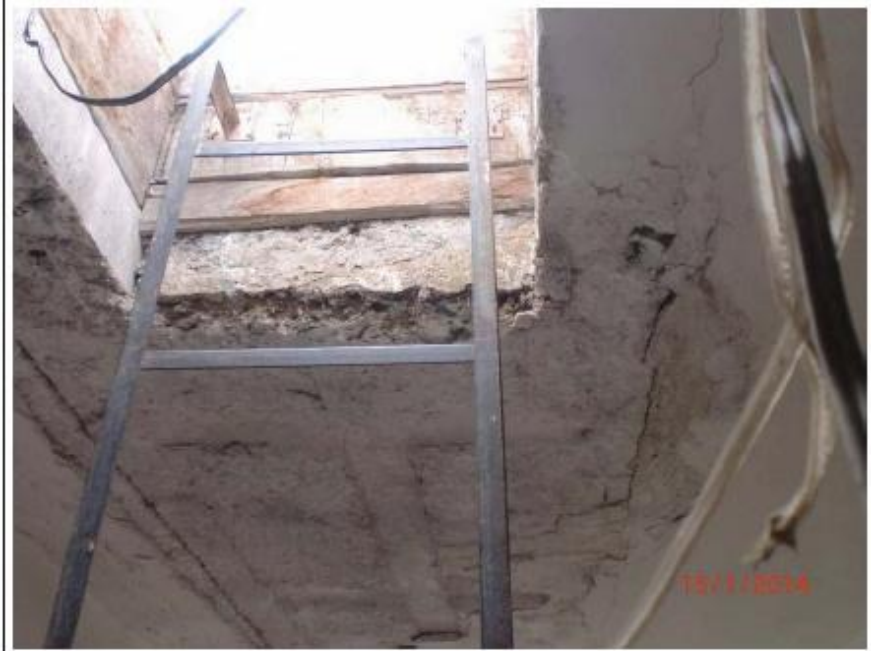
Main building 4. floor, Stairwell east side Roof hatch with concrete damage to the roof elements
