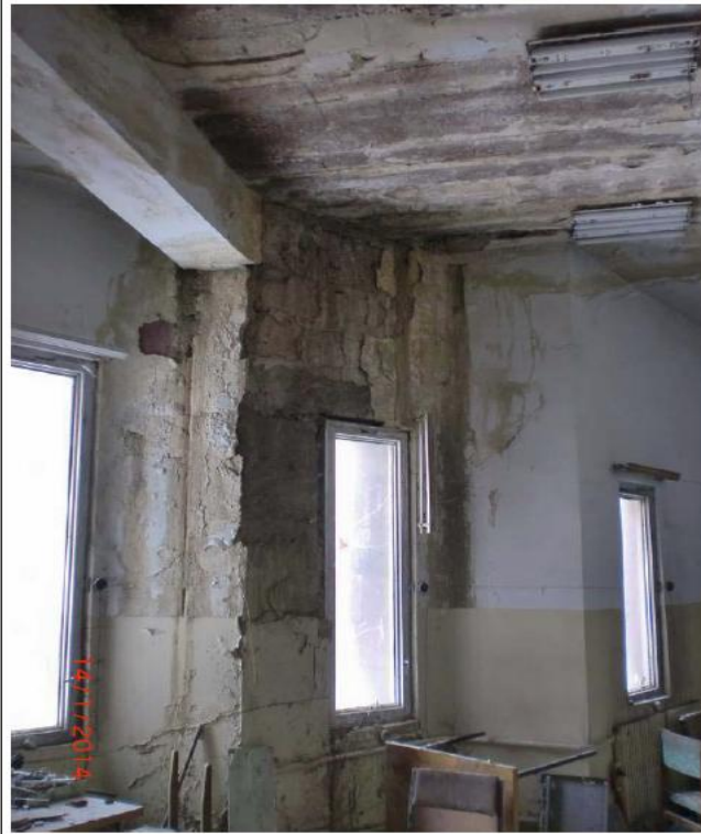
Extension 1. floor, Moisture damage and flaking on the ceiling and outer wall (Receiving Area 1)
