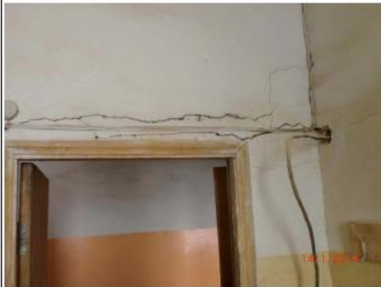
Main building 1. floor, Inner wall with subsidence on lintel of wood (Reception)
