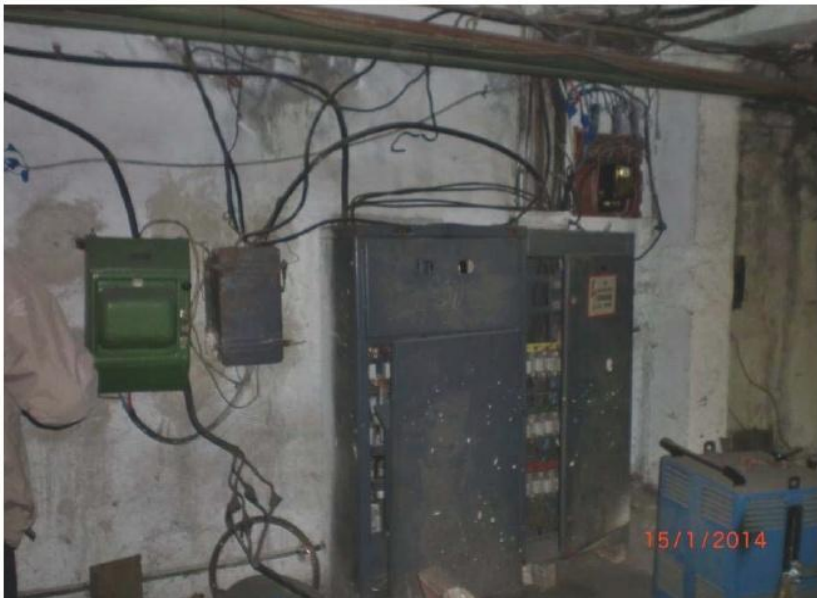
Main building basement, Electric service connection (Mass)
