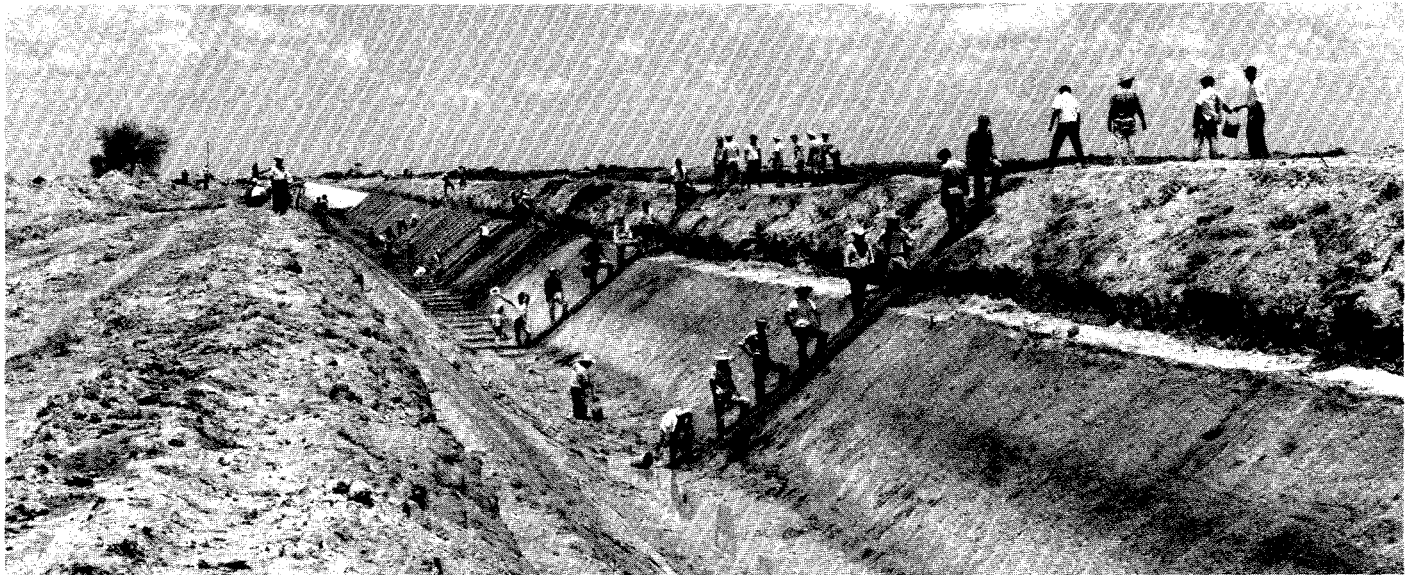
Building an irrigation canal near Empalme in the Rio Bravo region of northeast Mexico. The World Bank has made finance available to Mexico for the development of industry, electric power, transportation and agriculture.
