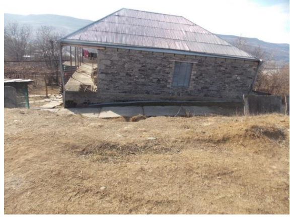
Damaged fence as a result of Jorjiashvili canal filtration
