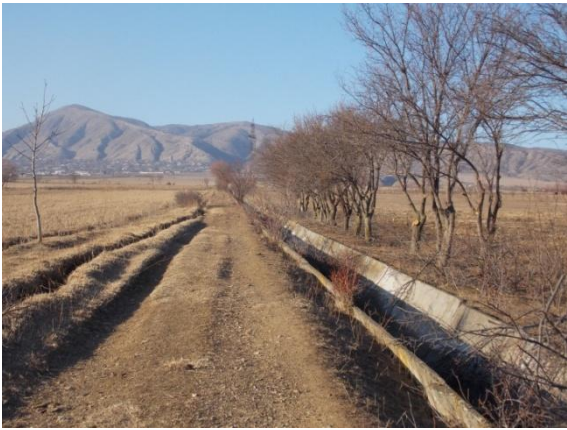
Parabolic inclined canal
