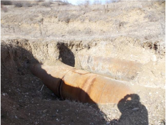
Damaged section of Bogvi inverted siphon
