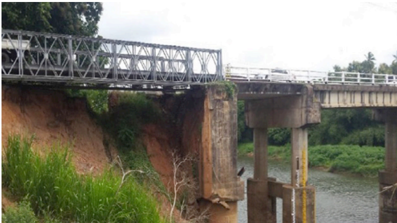
Figure C.13. Typical Damage to a Bridge Abutment caused by Flood Flow in Sri Lanka
