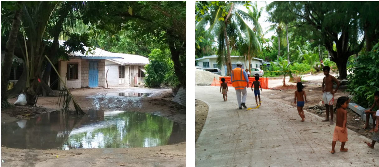
Figure C.9. Feeder Road on South Tarawa, Kiribati Before and After Construction of Geocell Pavements
