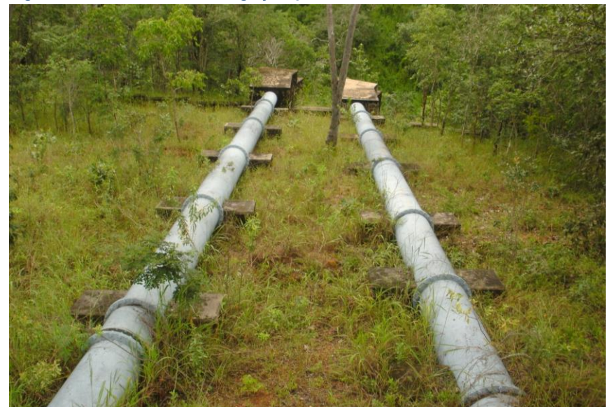
Figure 8. Penstock of an existing hydropower scheme.
