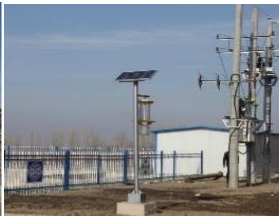
项目实施后机电设备及管理房 Electromechanical equipment and management room after project implementation
