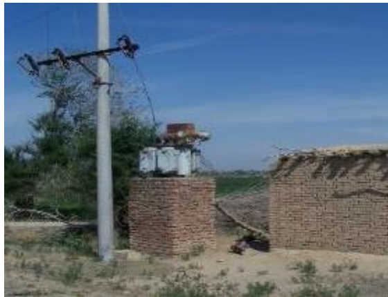
项目实施前机电设备及管理房 Electromechanical equipment and management room before project implementation
