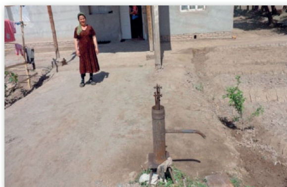
Photo 6. Hand pump in yard, Beruniy Raion, Karakalpakstan region
