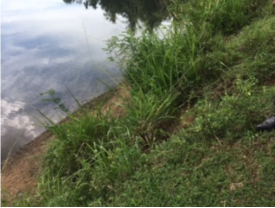
Example of embankment erosion
