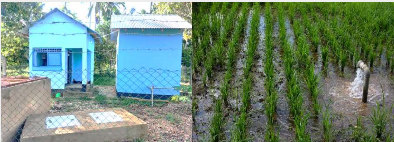
Pumping unit (left), individual plot (right) equipped with hydrant for watering at Koani scheme in Zanzibar (Source: Annual Reports)
