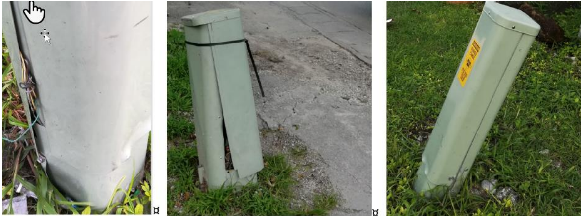
Figure 10 - Examples of Copper network condition in Majuro
