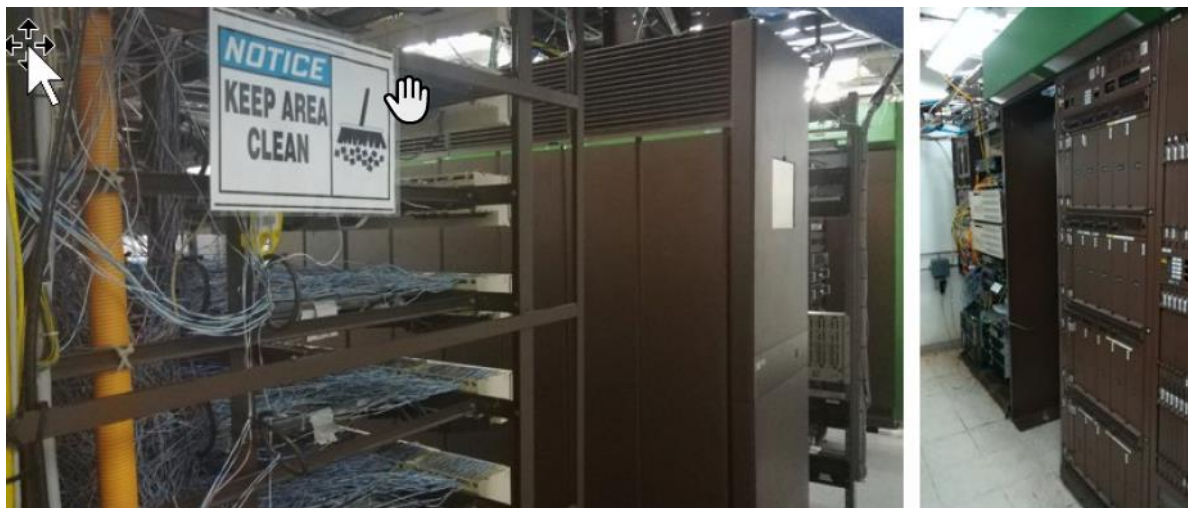
Figure 14 - Existing Nortel telephone exchange and equipment. The left is the copper termination in the main NTA building, the right is an example of the equipment in the remote sites of Airport and Laura.
