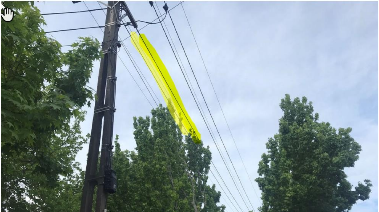
Figure 26 - Example of aerial deployment in New Zealand. Fiber cable highlighted in yellow. It is much closer to the power infrastructure than traditional deployments and the cable size and form is almost identical to the low voltage mains distribution network.. This allows a common path through any foliage and reduces the visual impact.
