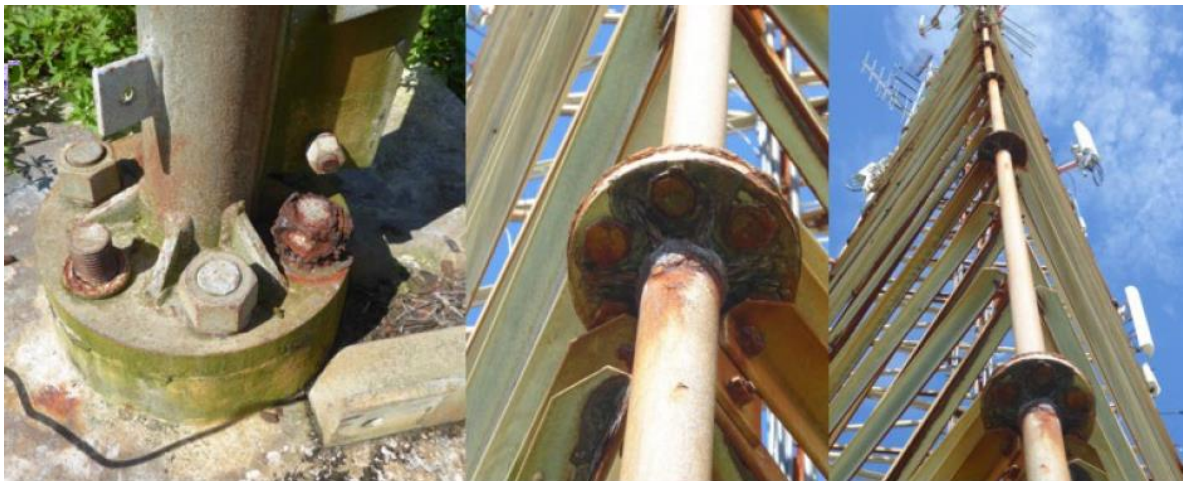
Figure 13 - Condition of Majuro Towers 2017/8
