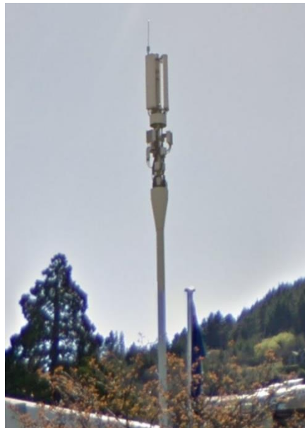
Figure 7 - Example of upgraded mobile tower in Queenstown NZ. Multiple frequencies have been added to provide Gigabit throughput.
