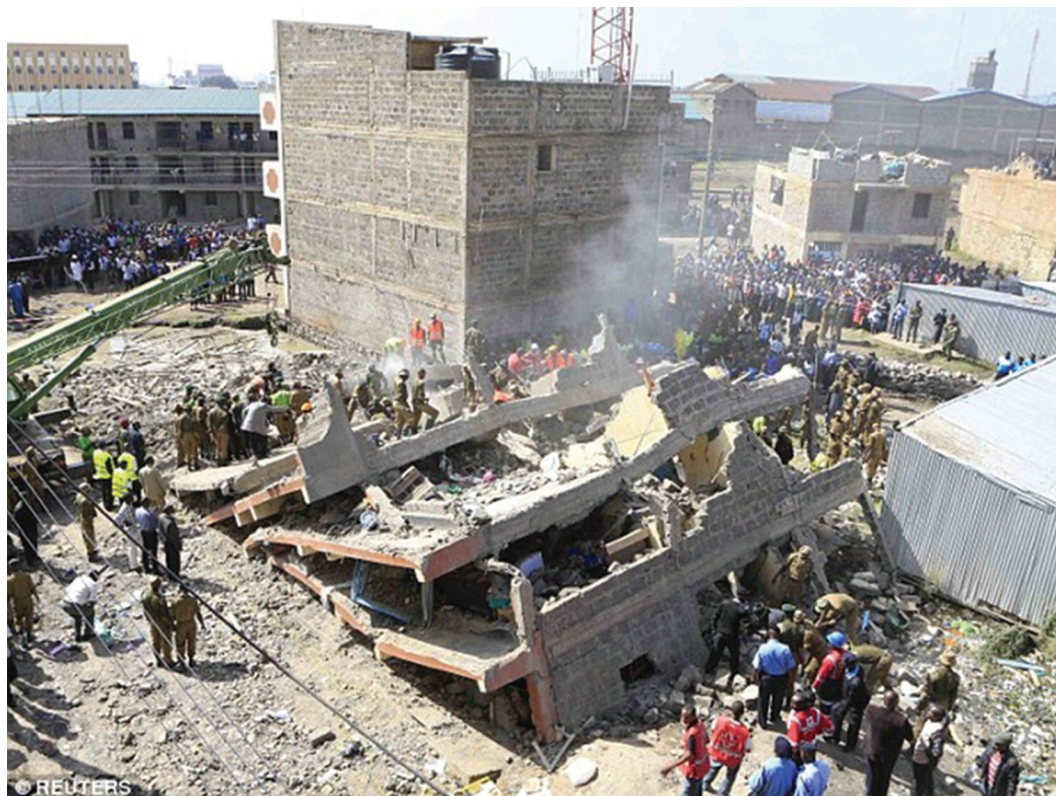
Figure 10: The case for development control—building codes are evaded and residential structures collapse and kill residents
