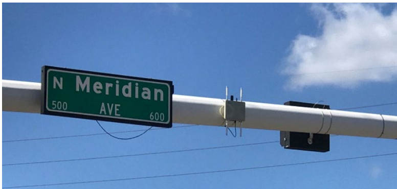
A. RSU INSTALLED ON MERIDIAN AVE (TAMPA, FLORIDA)
