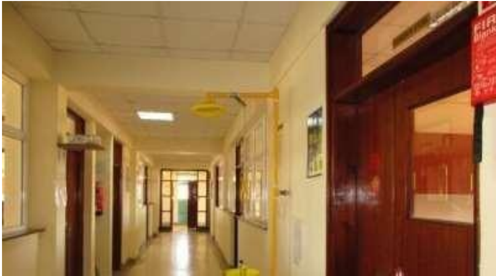
Plate 6: Face/Eye wash unit
