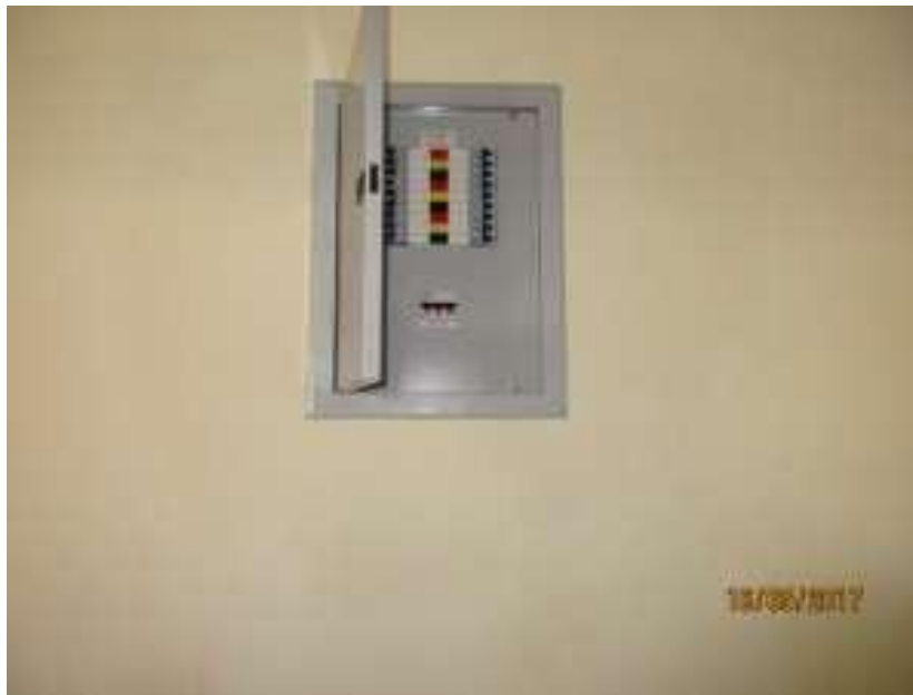
Plate 7: Functional Power Panel
