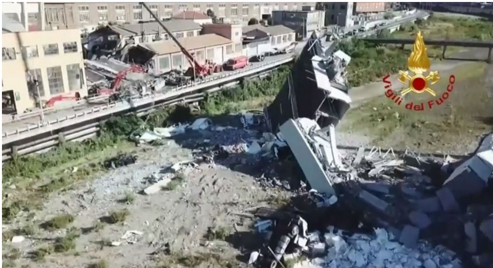
PHOTO 3.2 AERIAL PHOTO BY UAV, BRIDGE DEBRIS - GENOA, ITALY
