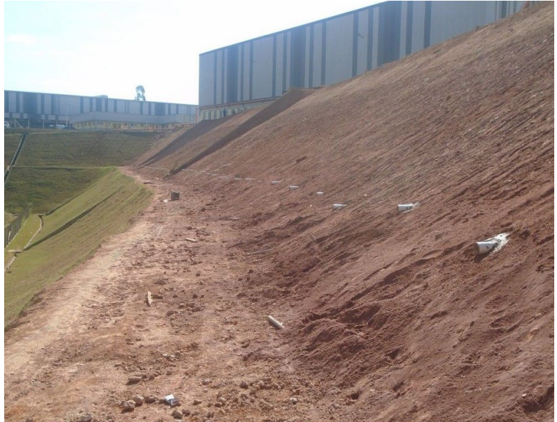
PHOTO 4.2 DEEP HORIZONTAL DRAINS
