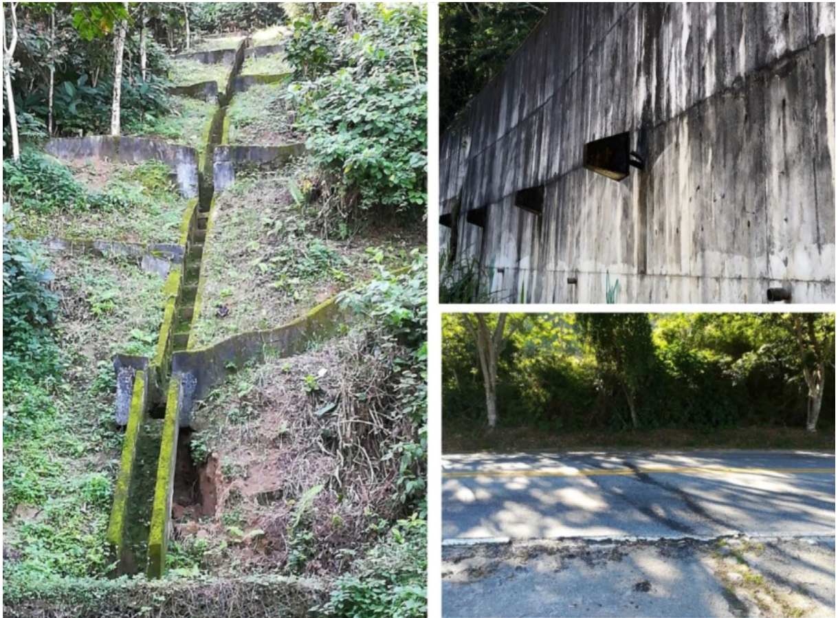
PHOTO 2.1 CRITICAL SPOTS IDENTIFIED DURING A FIELD VISIT, ANGRA DOS REIS, BRAZIL
